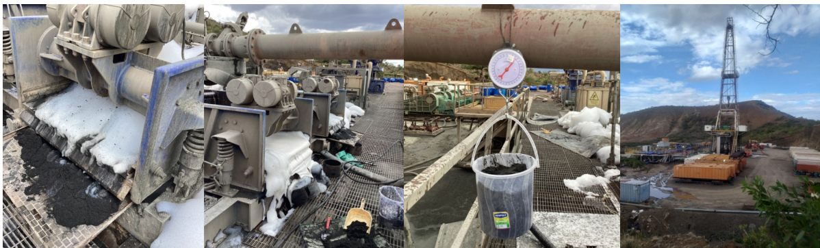
Figure 13: Data collection at well site during drilling at Paka geothermal field. The two images on the left show the shale shakers where the drill cuttings were collected. The third image shows the weighing of collected cuttings, and the rightmost image shows the drilling rig.
